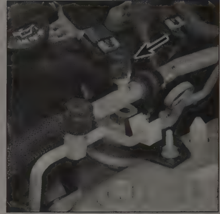
3.13 Location of the low-side charging port
