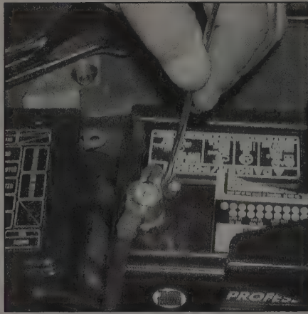
9.6b Removing a cable from the battery post with a wrench - sometimes a pair of special battery pliers are required for this procedure if corrosion has caused deterioration of the nut hex. Always remove the negative (-) cable first and hook it up last!
