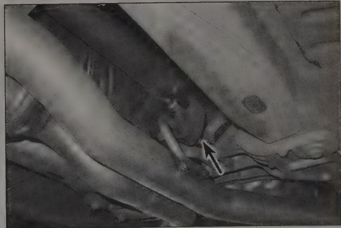
21.2 Be sure to check each exhaust system rubber hanger for damage
