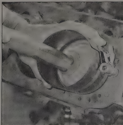
9.35 Use a plastic or wooden hammer handle to push the piston into the cylinder
